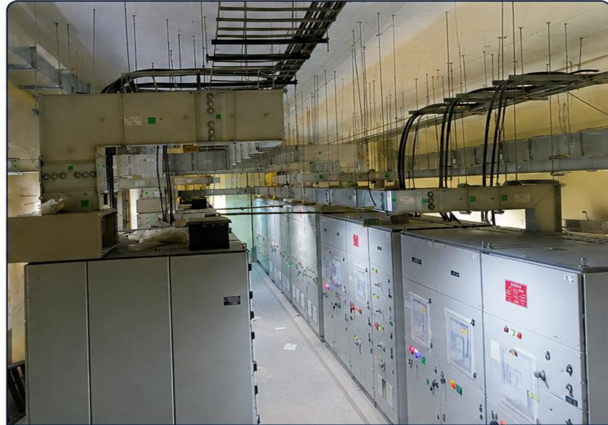
LT PANEL & BUS DUCT INSTALLATION
