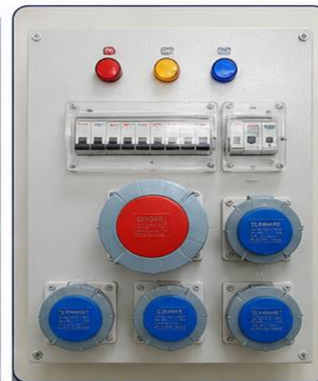
POWER DISTRIBUTION PANEL
